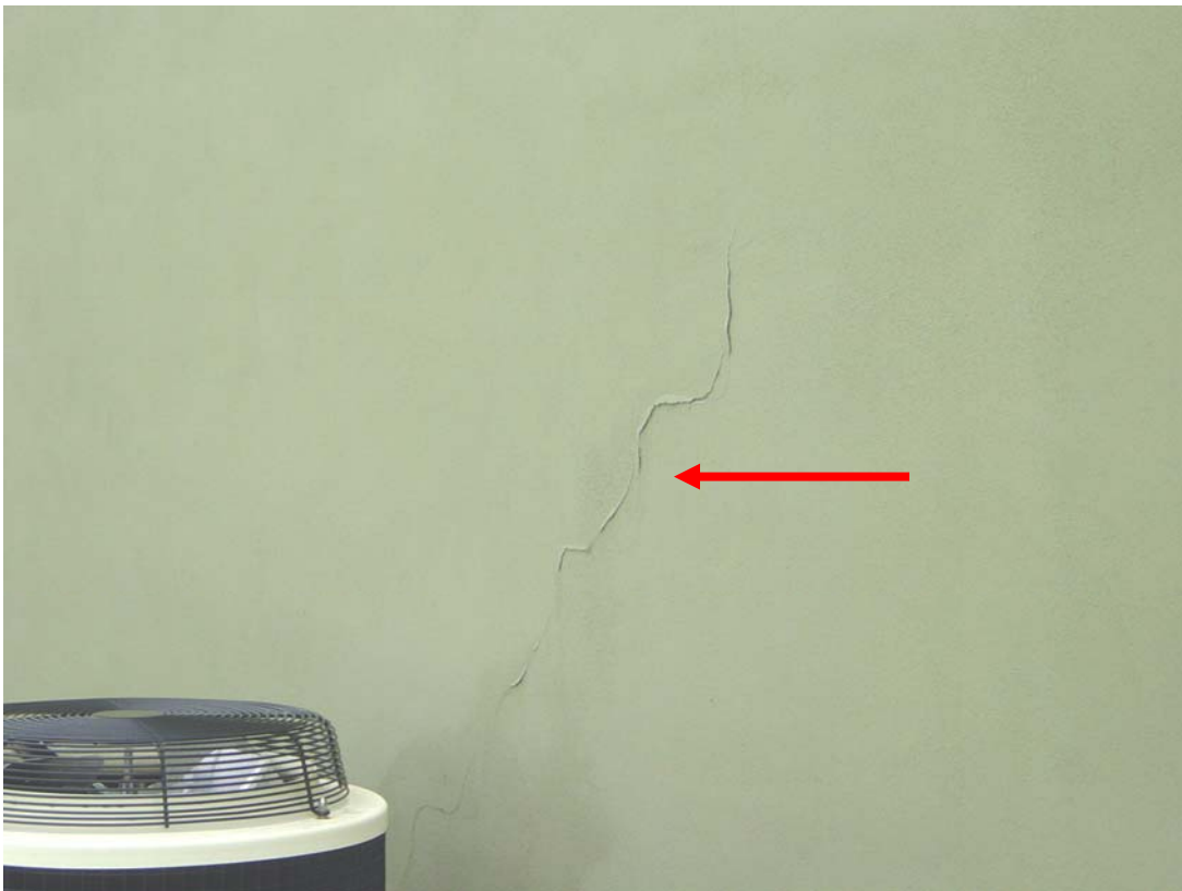
Stepped cracking on exterior wall from ground settlement
