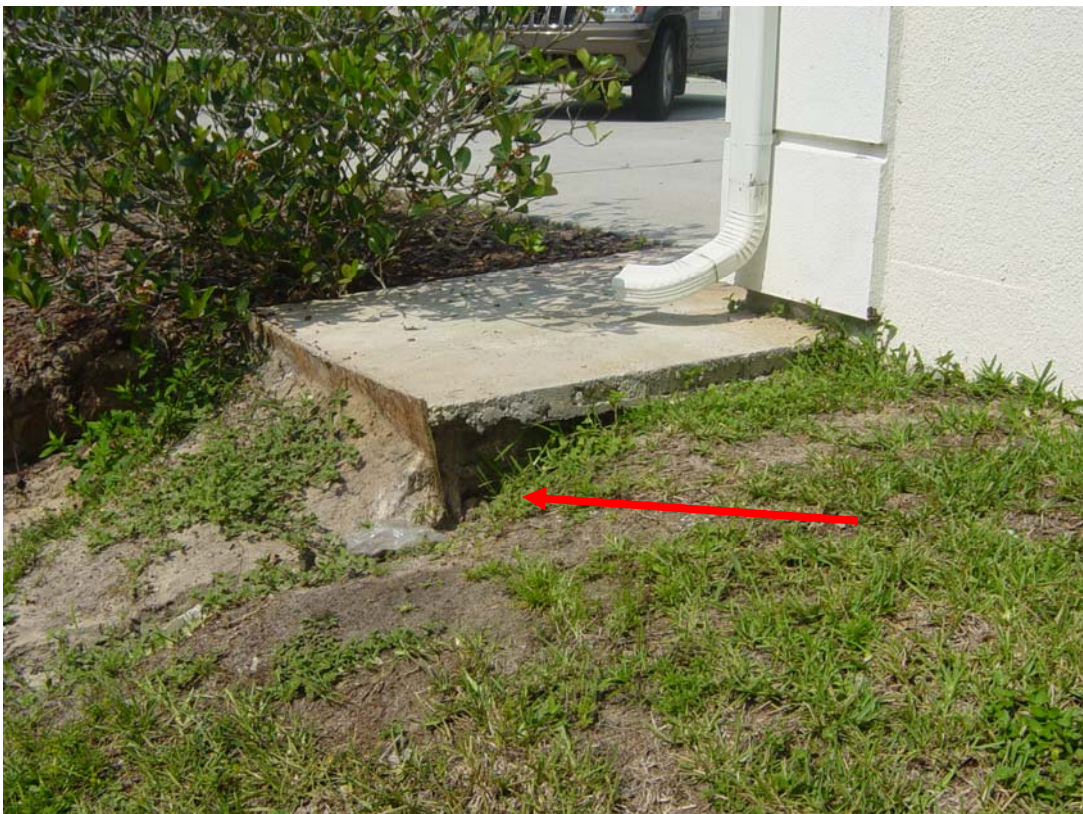
Soil erosion causing foundation failure
