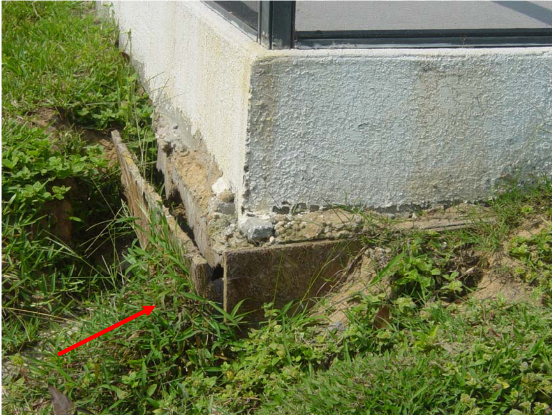
Soil erosion causing foundation failure
