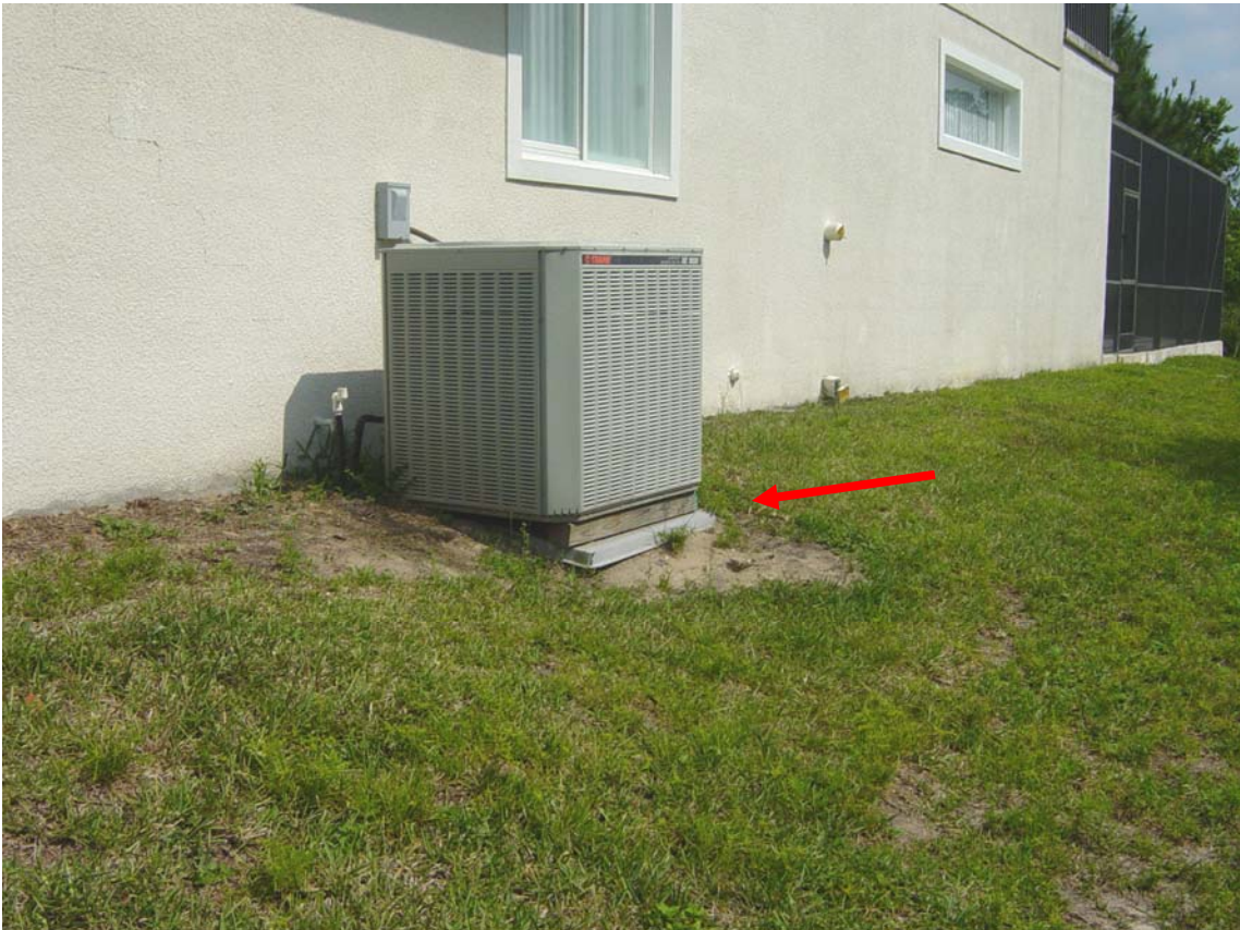
Soil erosion from poor grading causing the A/C unit to slip over. Packing timber keeping it level
