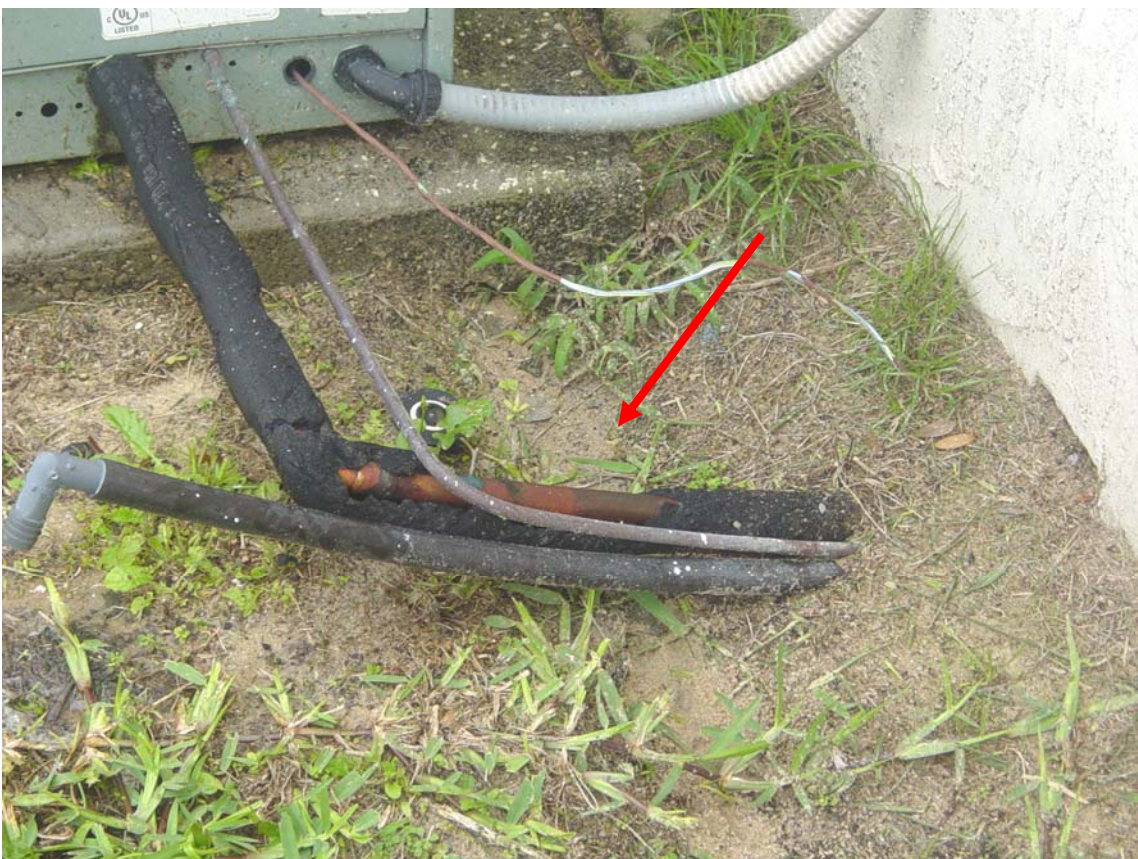
Damaged insulation on refrigerant lines.
