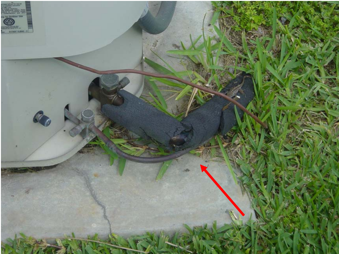
Damaged insulation on refrigerant lines.
