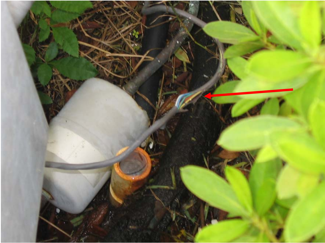
Damaged cables to A/C unit
