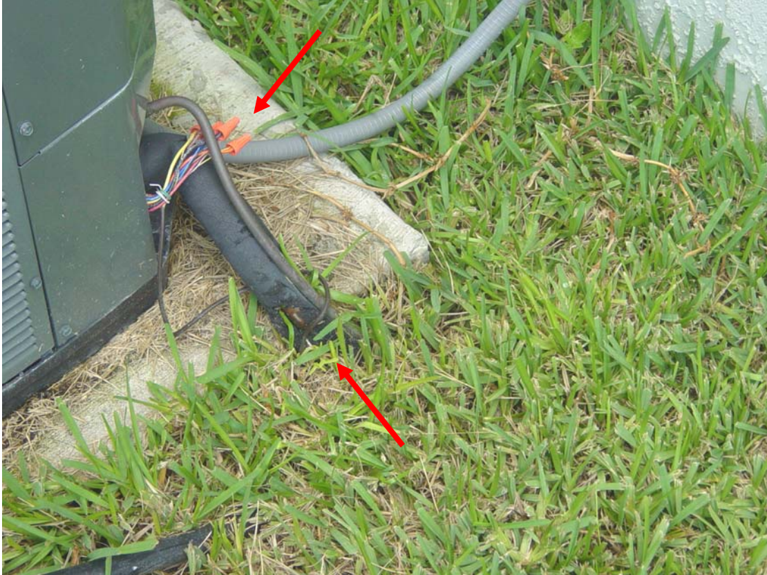
Exposed cables and damaged insulation on refrigerant lines.
