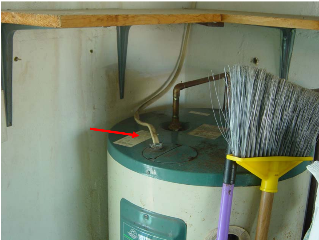
Exposed non armored cable above water heater
