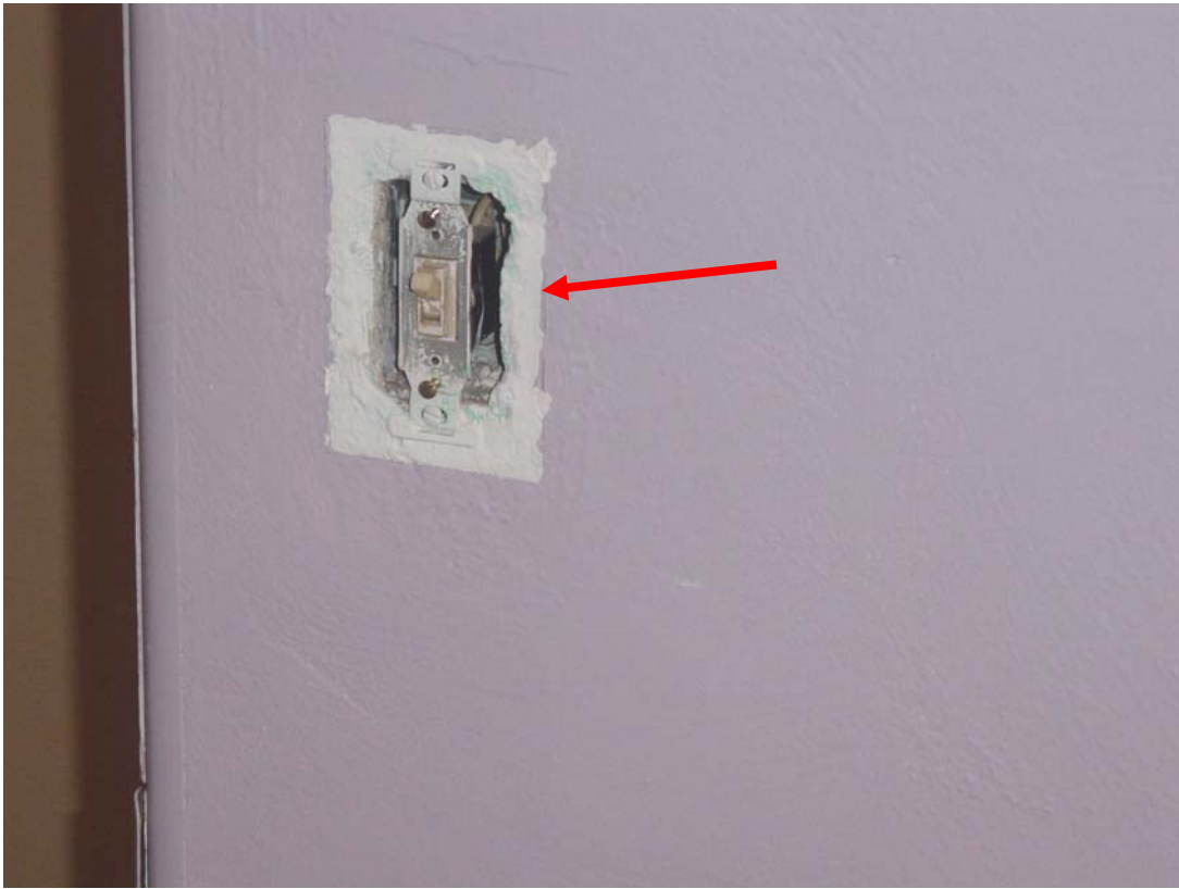
Missing cover plate from wall light switch
