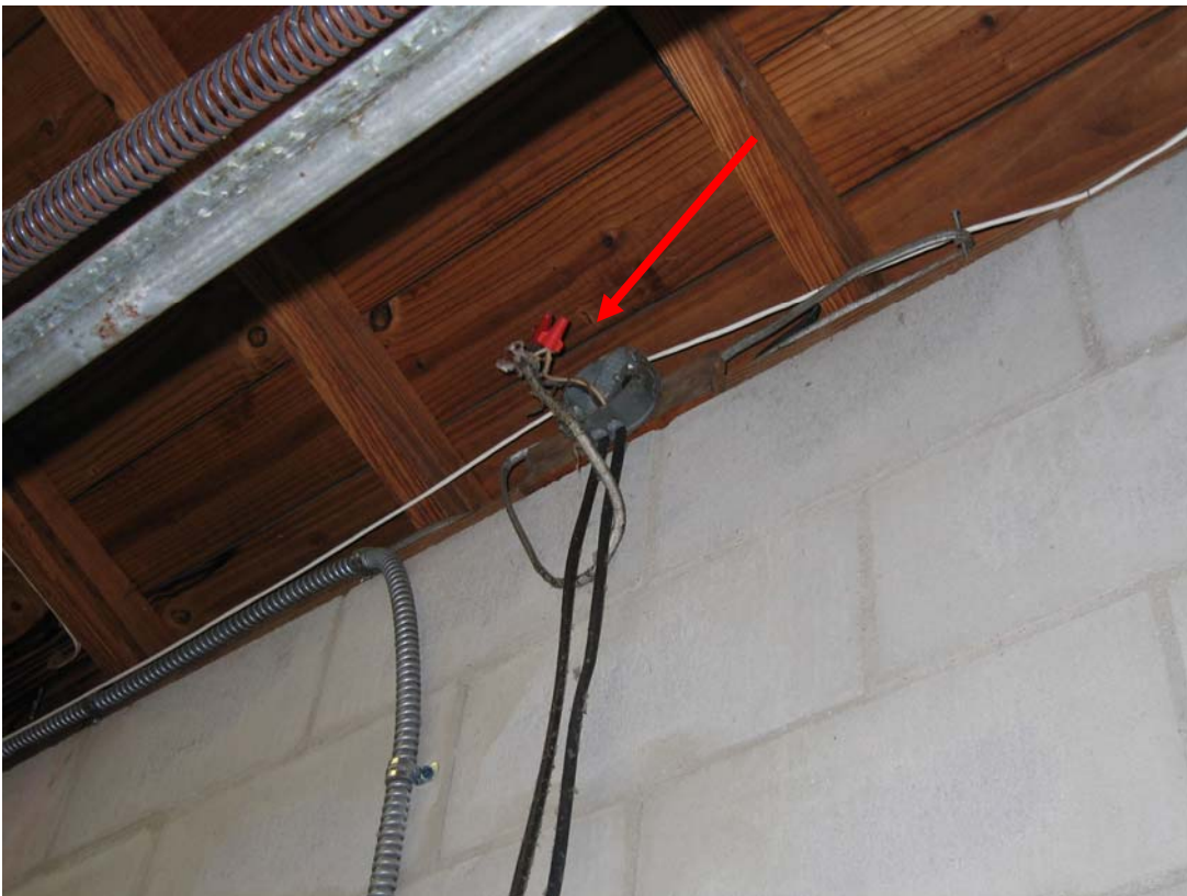
Exposed hanging live cables
