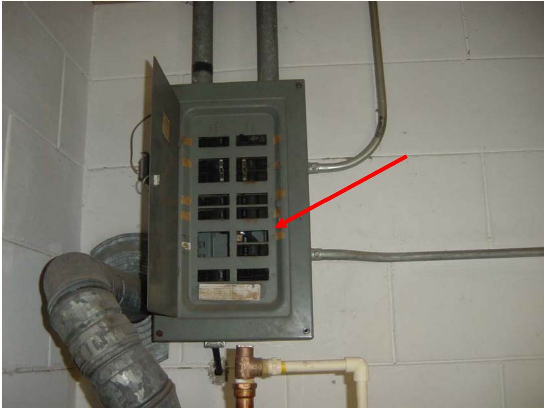
Missing breakers on service unit.
