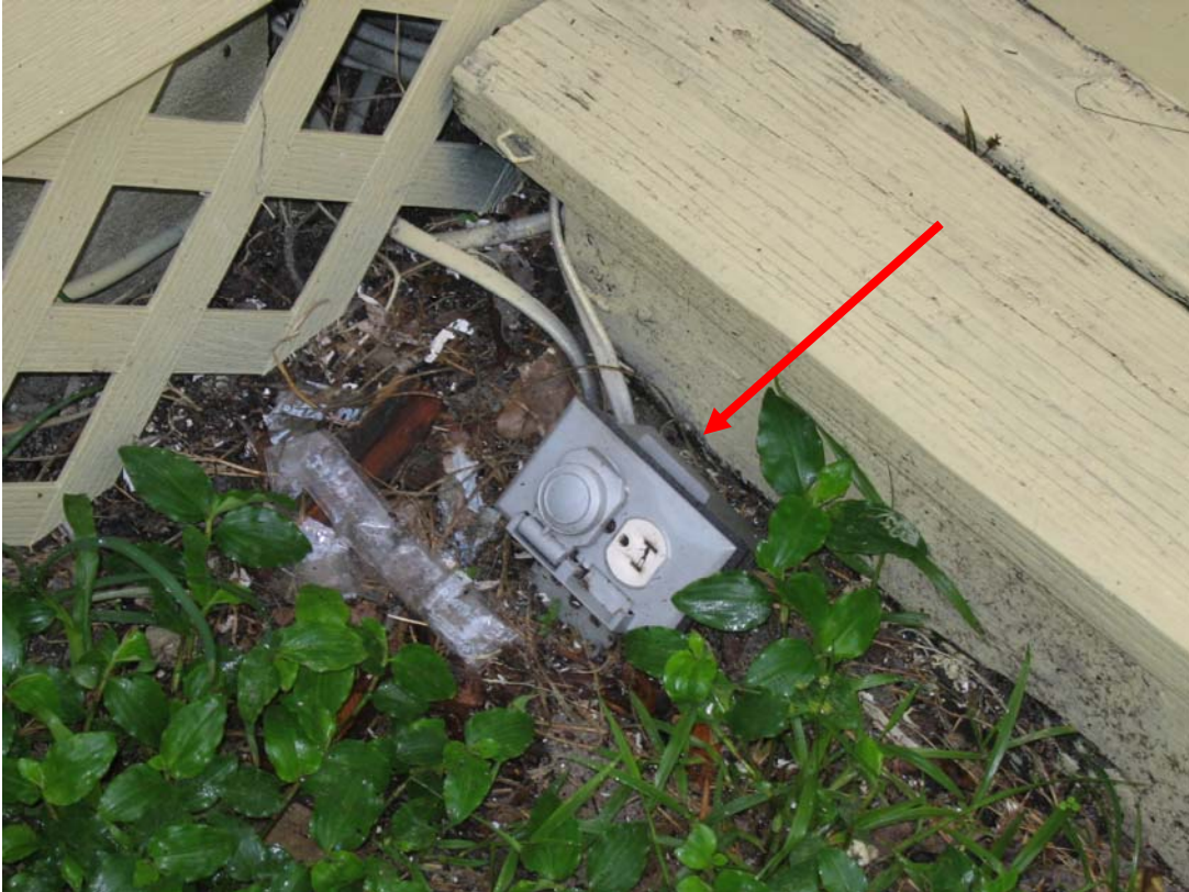
Buried electrical box in rear garden
